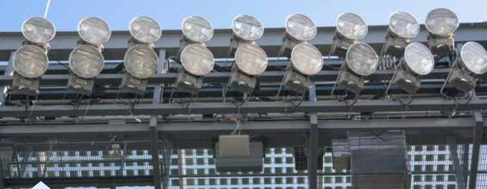
Photo shows Verizon Catwalk Distribution Antenna System (DAS).
