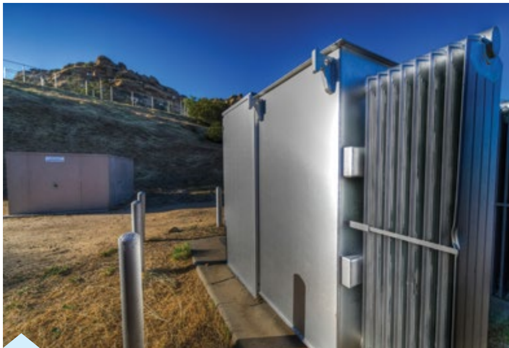
This is one of several in-park control units that accepts high voltage electric current from Southern California Edison Company and reduces it with in-park transformers to a low 120 volts. Larry LaCom/Summit Life photo.
