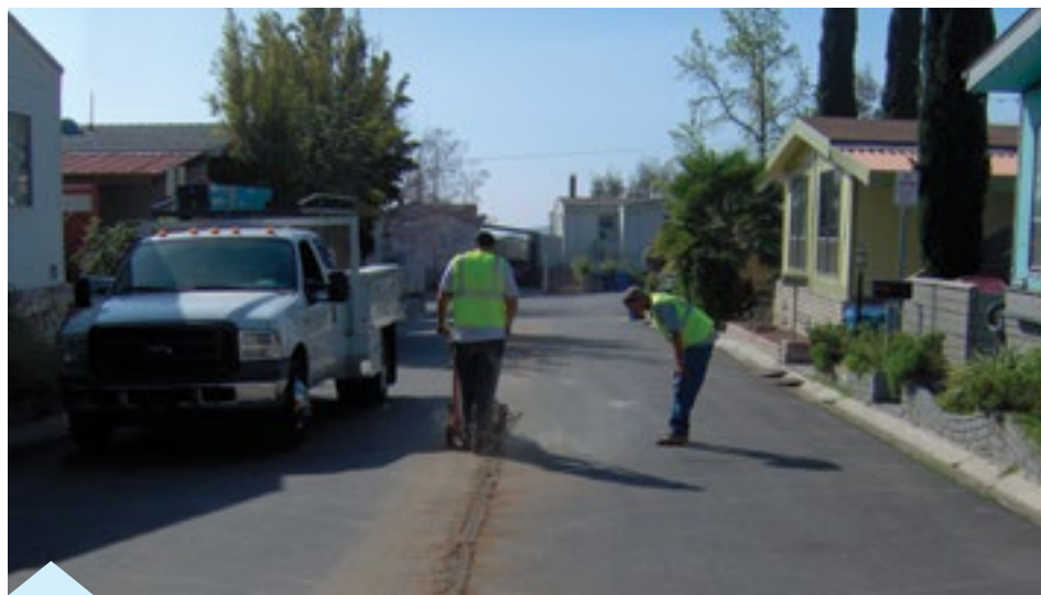
MAJOR SURGERY: workers prepare to slice-open middle of Club House Drive to install new electric cable. Driving down the trenched street covered with thin boards was only a part of the difficulties experienced by Summit residents during intermittent electrical outages.
